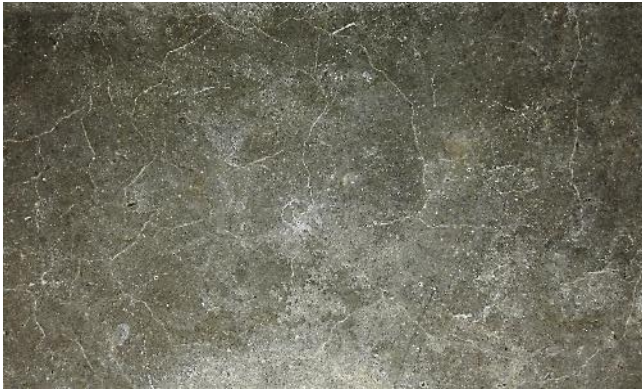
Figure 12. Example of cracking patterns of the specimens.
