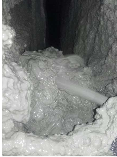
Figure 1: Detail of two-component injection in the annular void at the TBM launching chamber of SMP4 jobsite
